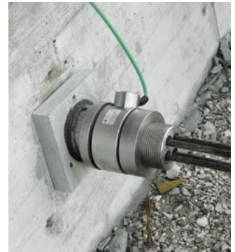
Fig. 2: HRL-4-1000 (4 strands) mounted on cable anchor
