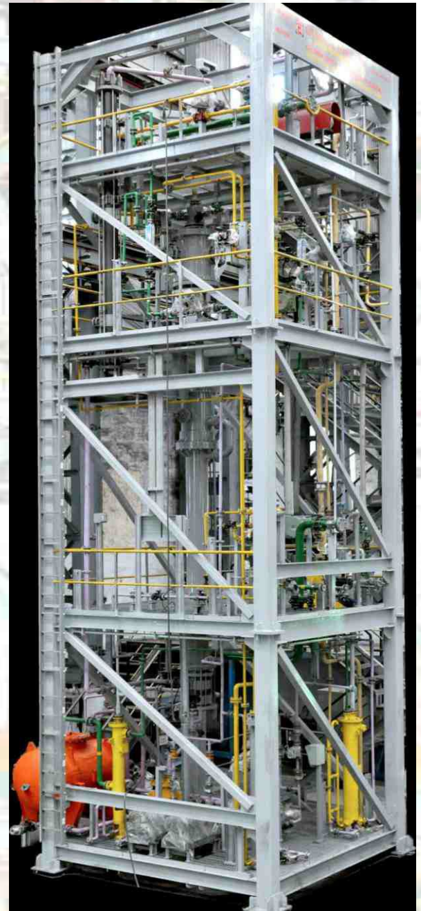
Skid mounted unit
